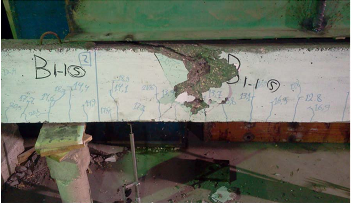
Photo (5) Failure of the tested beam {B1-1 (S)}.
