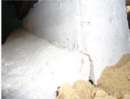
Photo (5): Failure Shape of Folded Strip Footing.
