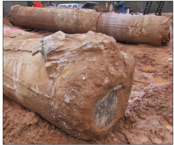
Fig.7. Post-grouted pile showing grout flowing up the side of the pile, Brown et al., (2010) [18].
